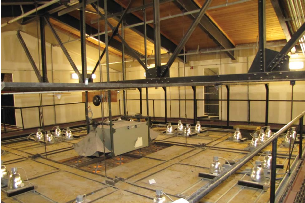
Figure ES05: House skylight attic showing top of bronze ceiling laylight with speaker cluster at the center. A perimeter catwalk provides access.
