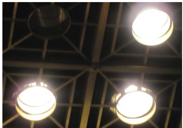
Figure 21: Light leaks / misalignment of downlights
