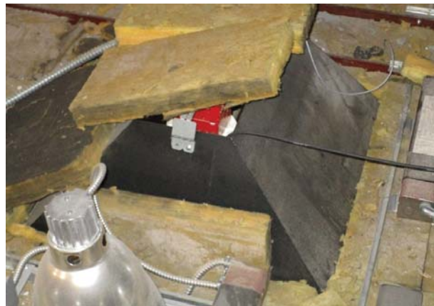
Figure 23: Smoke detector location in skylight attic
