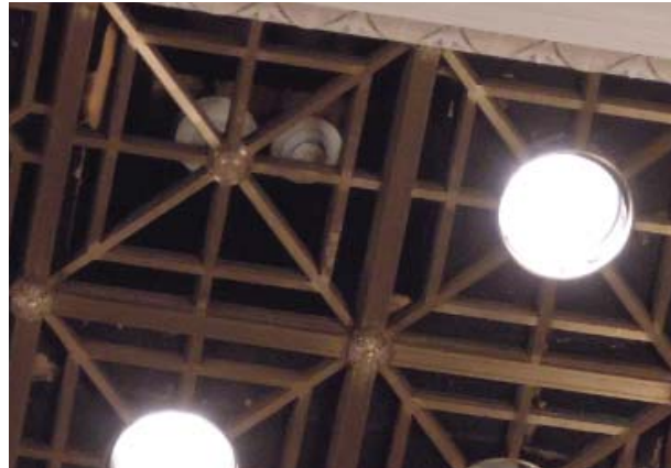
Figure 22: Smoke and heat detectors from Chamber floor
